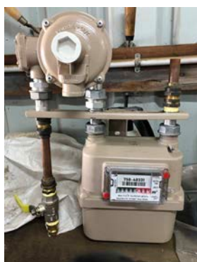
Domestic gas meter
