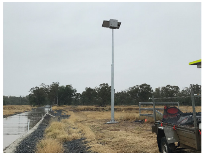
Above - New camera at Ashburns Road, Eastern Diversion Channel causeway.
