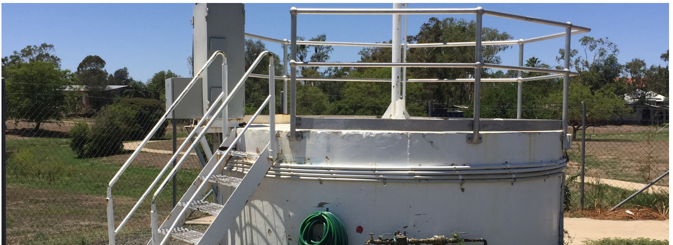
Roma's Sewage Pump Station.
