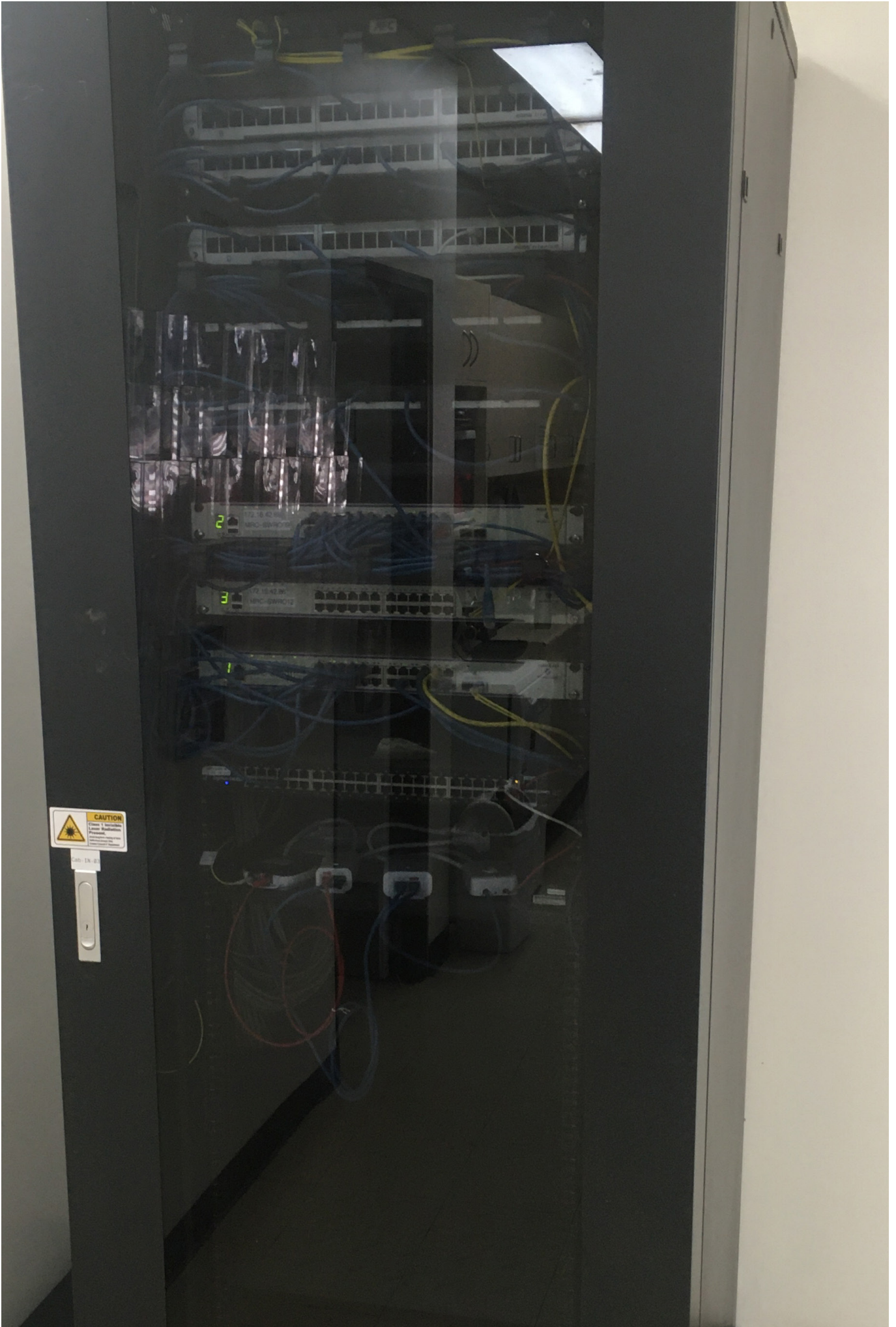
IT server at Council's Roma Infrastructure Depot
