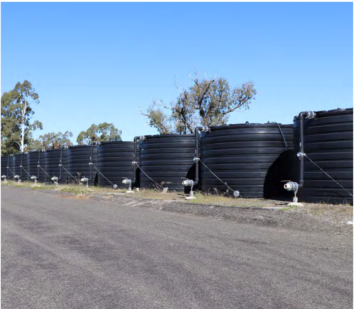
Roma Sewerage Treatment Plant
