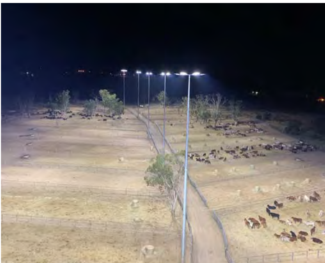
New lighting in operation at Roma Saleyards
