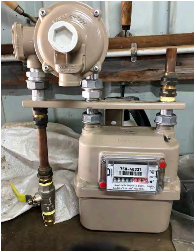
Domestic gas meter
