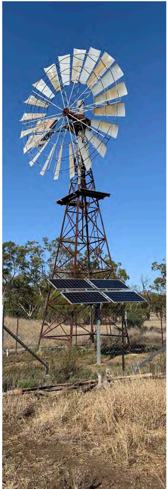
Capital works - Pegleg water facility
