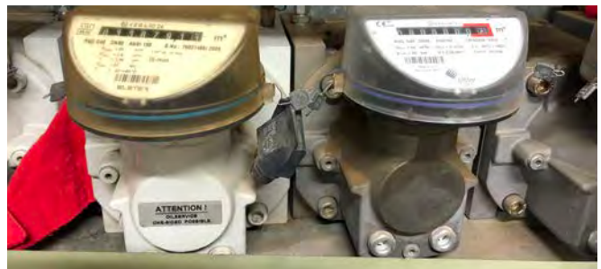
Commercial gas meter
