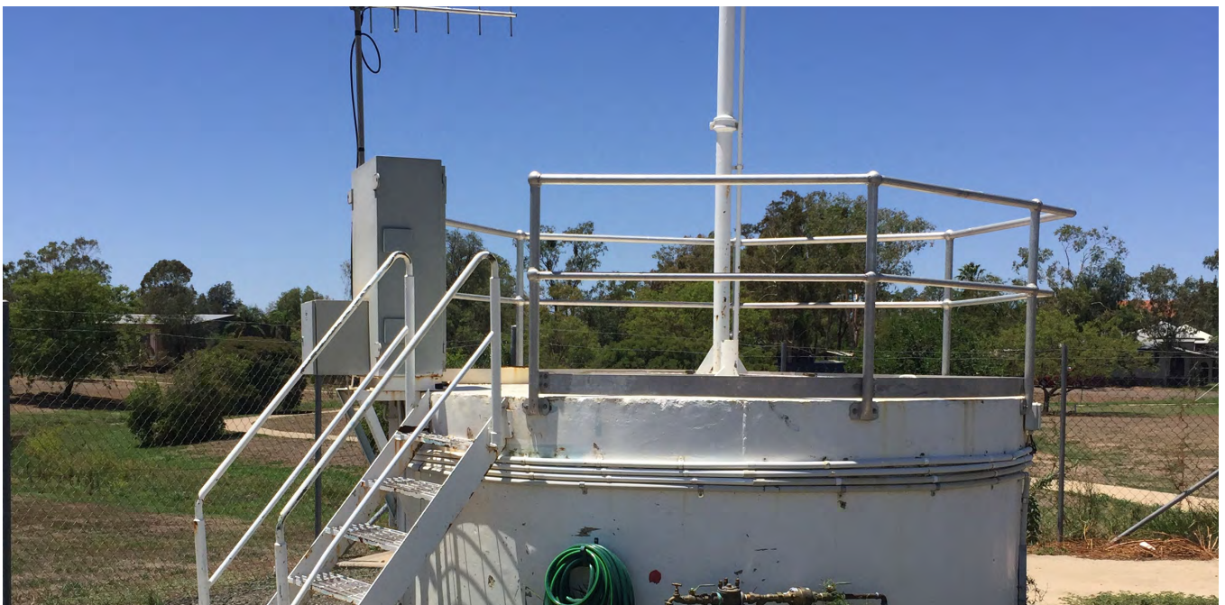
Roma's Sewage Pump Station.
