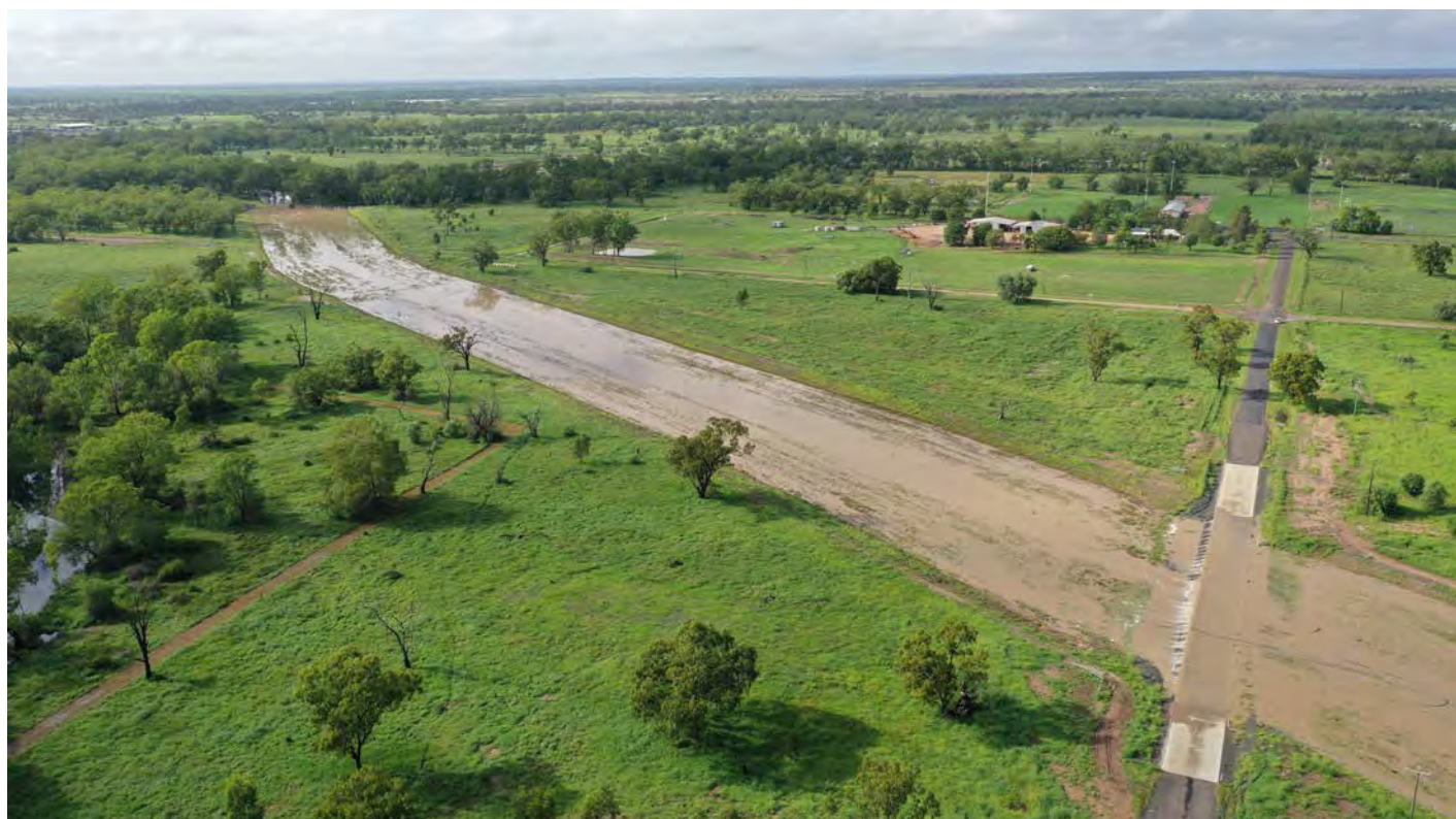
Eastern Diversion Channel - part of the Stage 2A Flood Mitigation Project, Roma.
