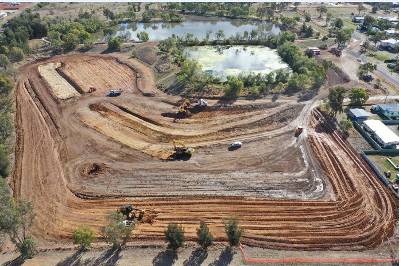
Stage 2b Roma Flood Mitigation Project - Railway Dam. This project was funded through the Queensland Government's Building our Regions Program and the Maranoa Regional Council.
