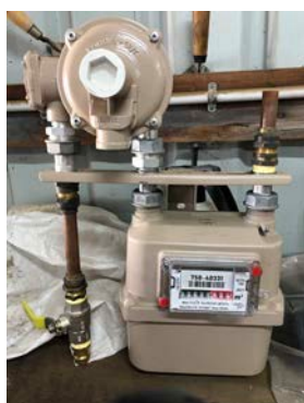
Domestic gas meter
