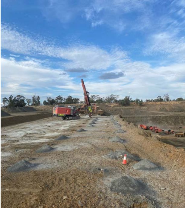
Preparing for a blast at the Roma Quarry for aggregates and subbase
