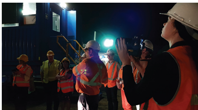
Communications Officer - Infrastructure Services Sophie Kluckhohn taking photos of key milestones at the Roma Airport Overlay Project (night time works).
