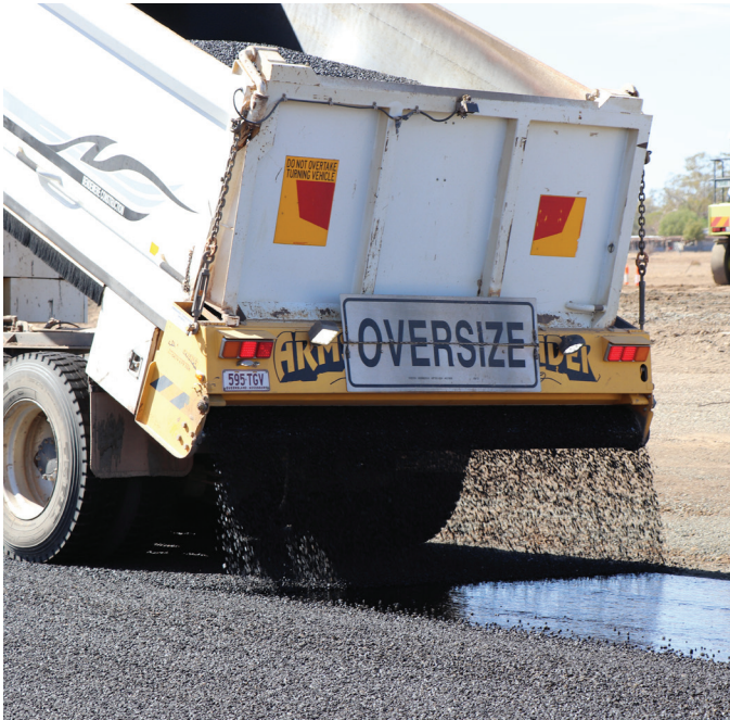
Bitumen surfacing works - Ivy Street, Roma. The Ivy Street project used a considerable volume of material from the quarry, including roadbase, bitumen sealing aggregates, concrete aggregates and drainage rock.
