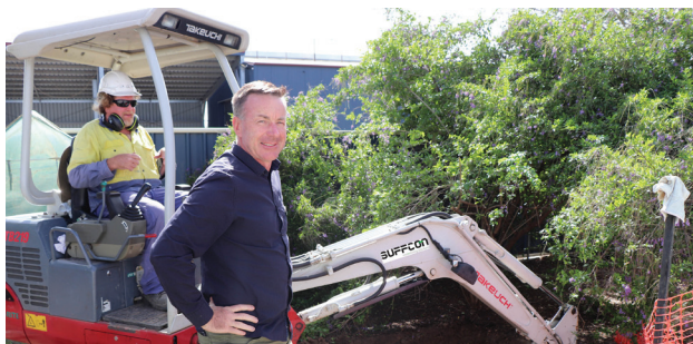
Cr David Scheffe, Portfolio Chair for Utilities, viewing the site of the sewer relining works with local contractor worker, Suffcon Pty Ltd.
