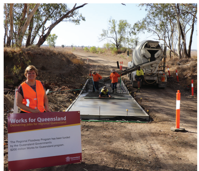
Cr Janelle Stanford views the works being undertaken on Gunnewin East Road - part of the Regional Floodway Program.
