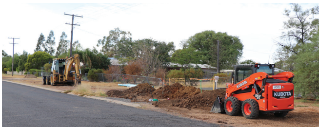
Golf Links Subdivision Fire Flow Augmentation, Corfe Road, Roma - funded by the Queensland Government's $200 million Works for Queensland program.
