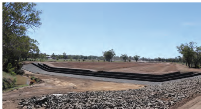
Works on Stage 2A flood mitigation during the year (including Eastern Diversion Channel (above) and an extension to the Stage 1 levee referred to as the 'Western Levee').
