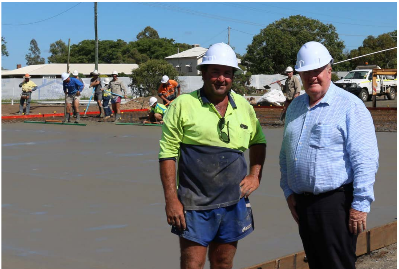
Contractor Brett Pollock and Cr Peter Flynn inspecting works at the Maranoa Netball Precinct.
